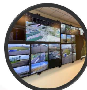
Central Control Room ZBR
