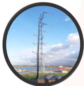
Radio Technology ROIP Antennas
